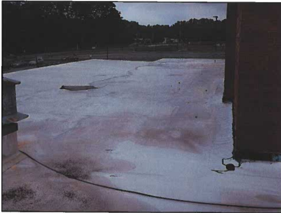
Photo 25: Ponding water on the lower roof, right side of the building.
