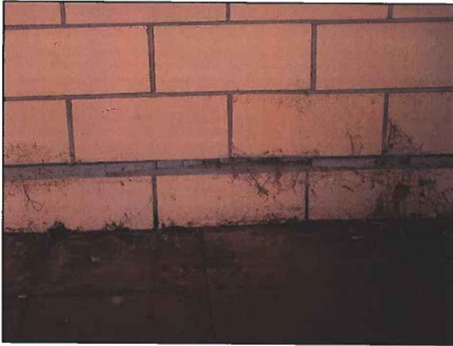
Photo 19: Open Joint in wall tile finish at rear of Gym space
