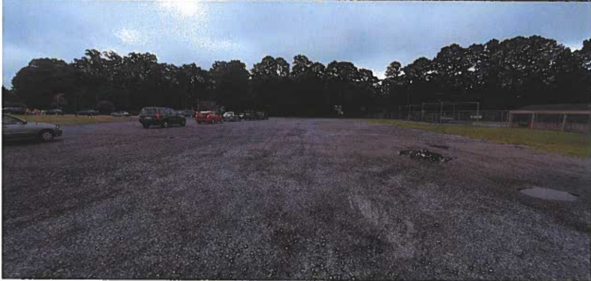
The existing gravel lot is heavily worn and eroded. This lot should be paved with asphalt or resurfaced with new gravel to flatten the surface and remove potholes.
