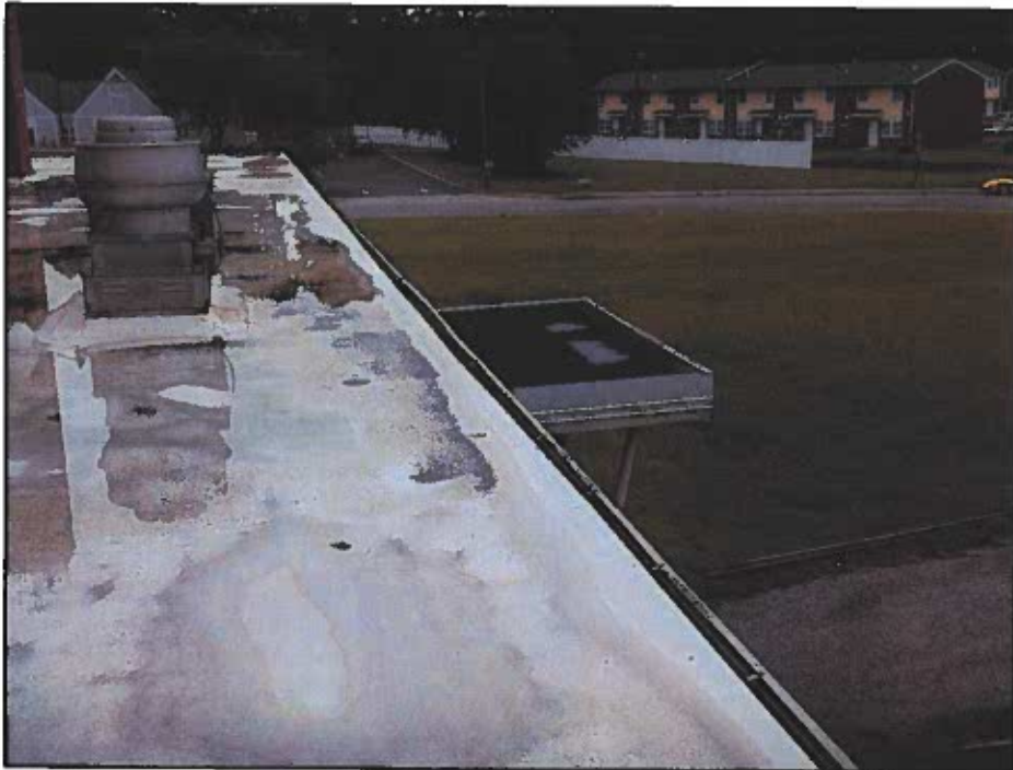
Photo 26: Ponding water on the lower roof, right side of the building.
