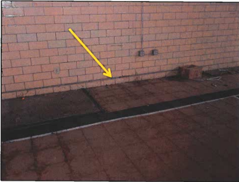
Photo 20: Open Joint in wall tile finish at rear of Gym space
