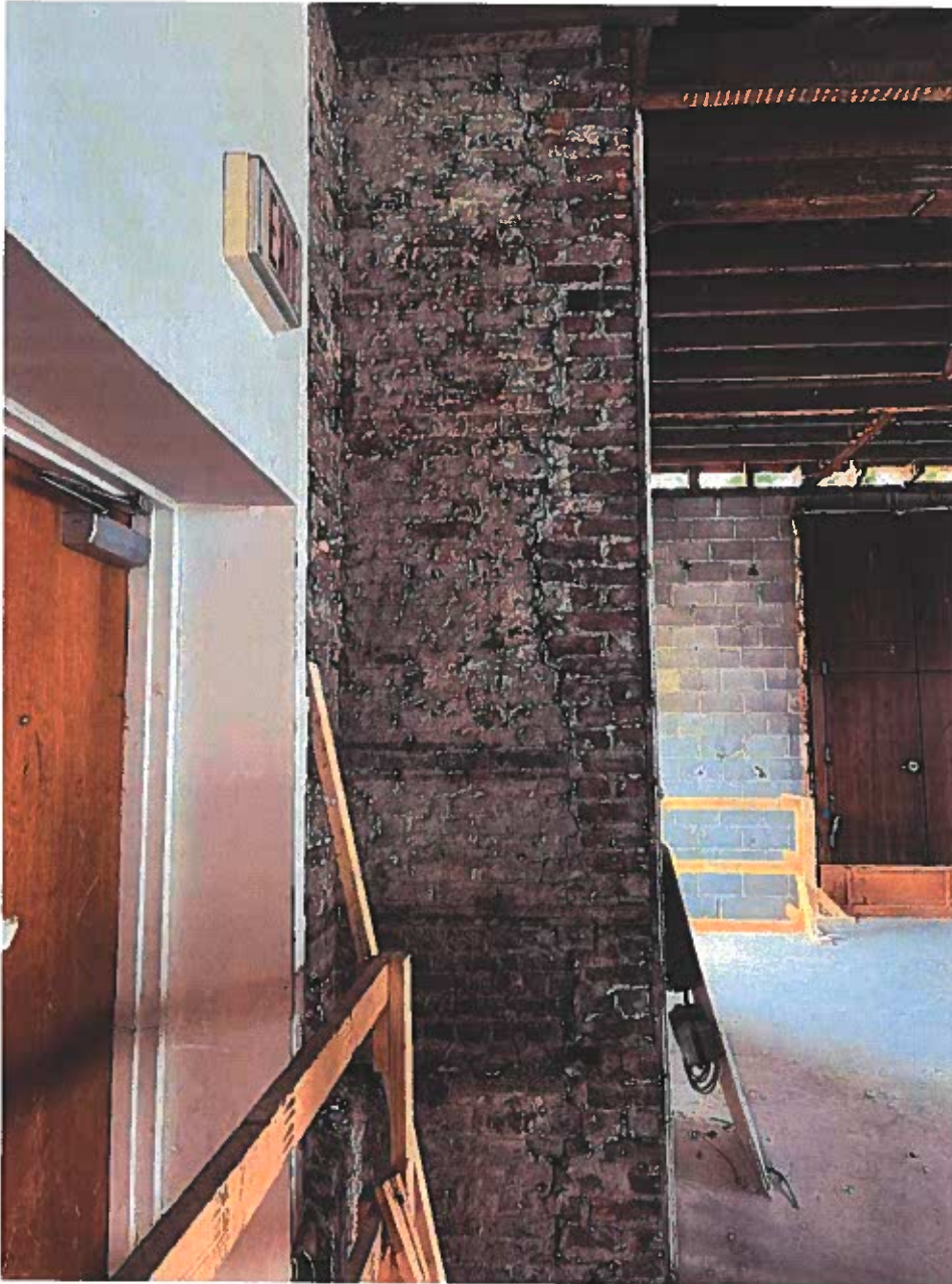
Photograph 3: crack in existing brick masonry wall
