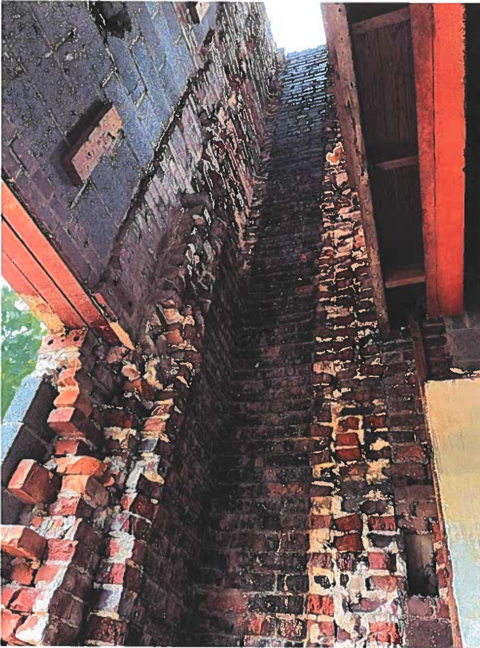
Photograph 1: Damaged brick in north east corner of existing building
