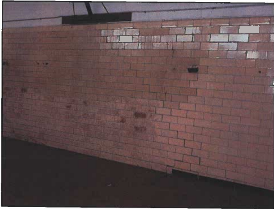
Photo 21: Cracks in the wall tile
