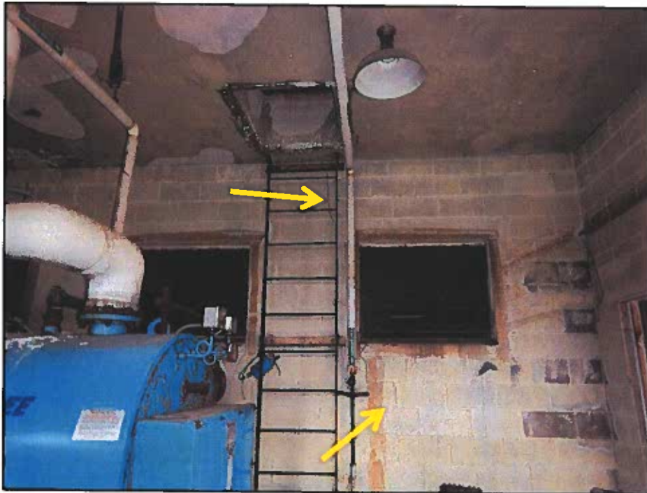
Photo 10: Large cracks at the roof access wall. This wall is an interior wall to the conditioned space on the right side of the building
