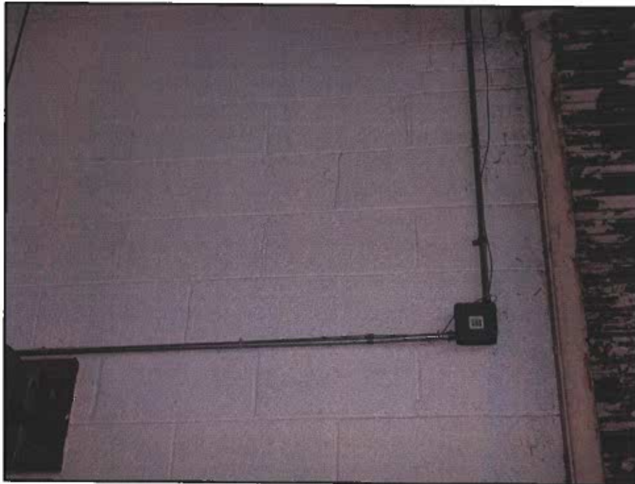
Photo 22: CMU Cracks at rear
