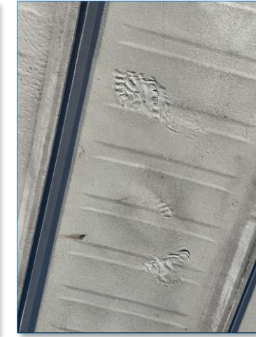
PREVIOUS COATING IS STARTING TO DETERIORATE THROUGHOUT THE FIELD
