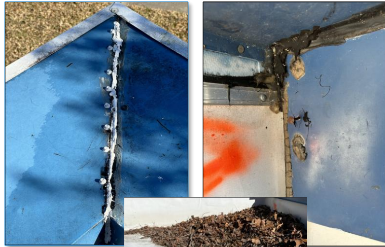
IMPROPER METAL DETAIL
