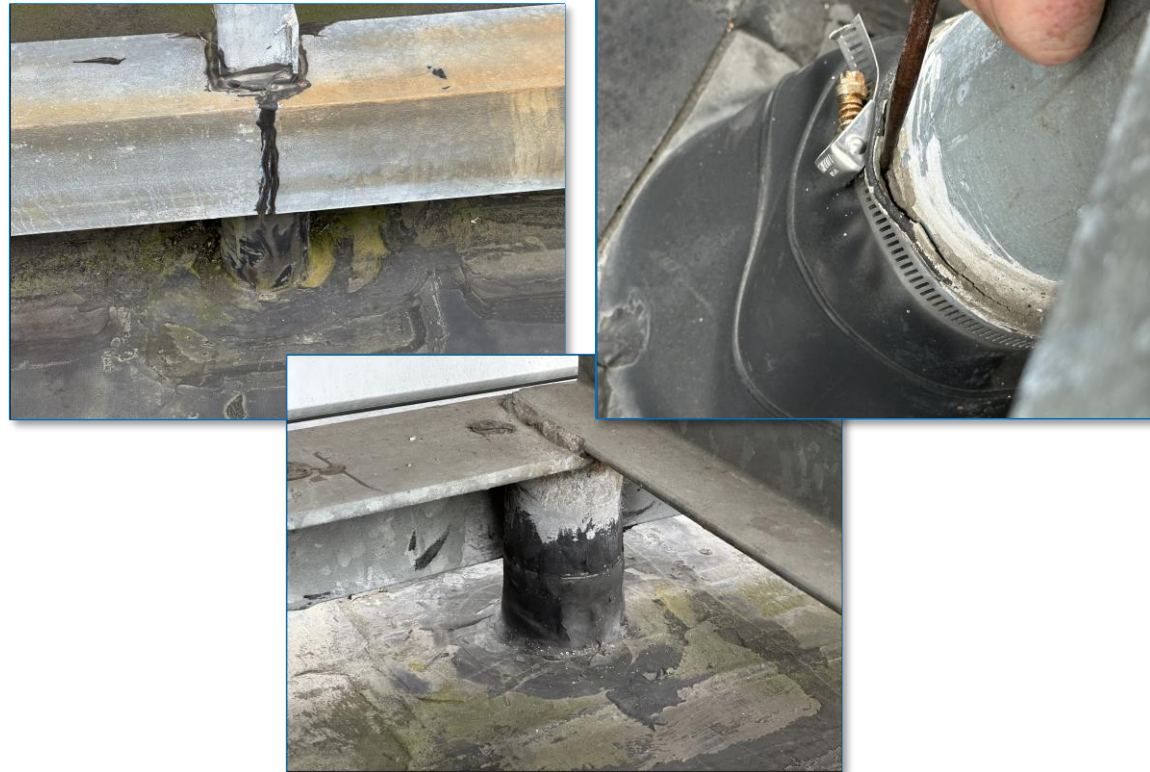
SEALANT HAS DETERIORATED. THE LOCATION OF POSSIBLE WATER INTRUSION AND LEAKS
