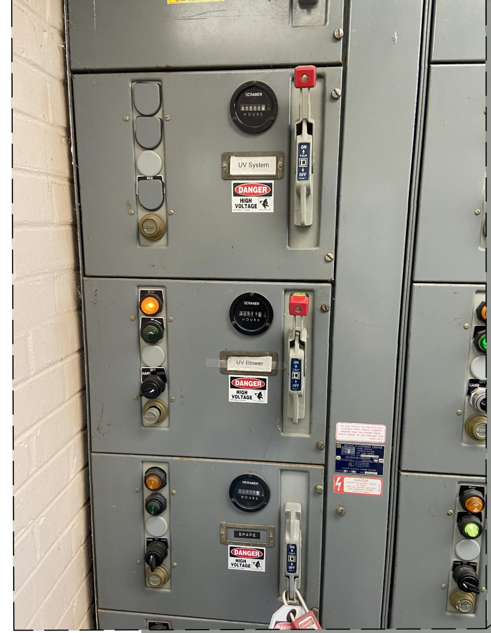
EXISTING BUCKETS IN MOTOR CONTROL CENTER (MCC) TO REMAIN. INSPECT EXISTING UV TREATMENT SYSTEM FEEDER FUSES AND WIRING IN MCC TO ENSURE THEY ARE IN GOOD CONDITION FOR REUSE.
